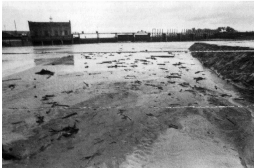
FIGURE 18.17 Spencer Dam on Niobrara River, Nebraska. View looking downstream across sand sediment deposits being scoured from the empty pool ( G. Morris ).
