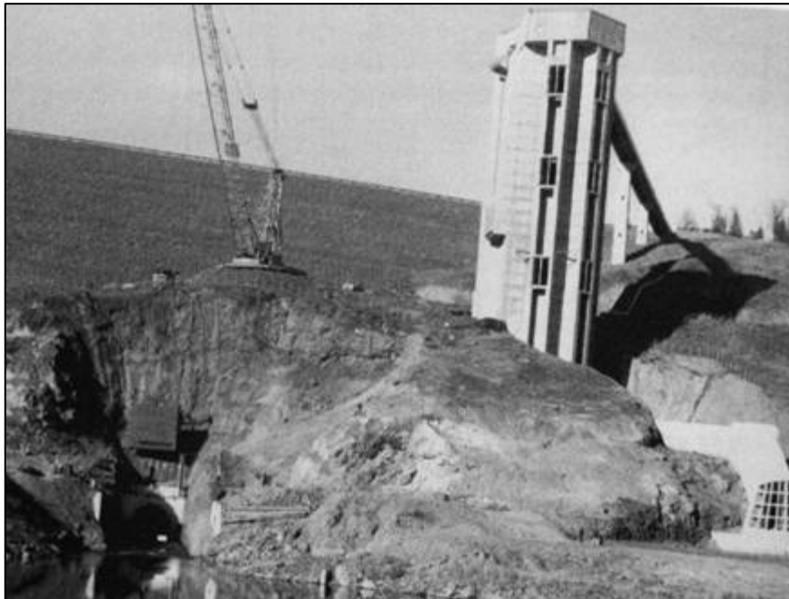
FIGURE 4.7 Outlet structures at Lost Creek Lake, Oregon. The Low-level outlet is on the left of the photo, and the selective withdrawal tower and the turbidity conduit connected to its base are visible on the right. (Courtesy U.S. Army Corps of Engineers)
