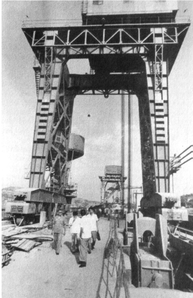
FIGURE 24.5 Vertical sluice gate (right fore ground) and gantry for gate placement. (G. Morris).
