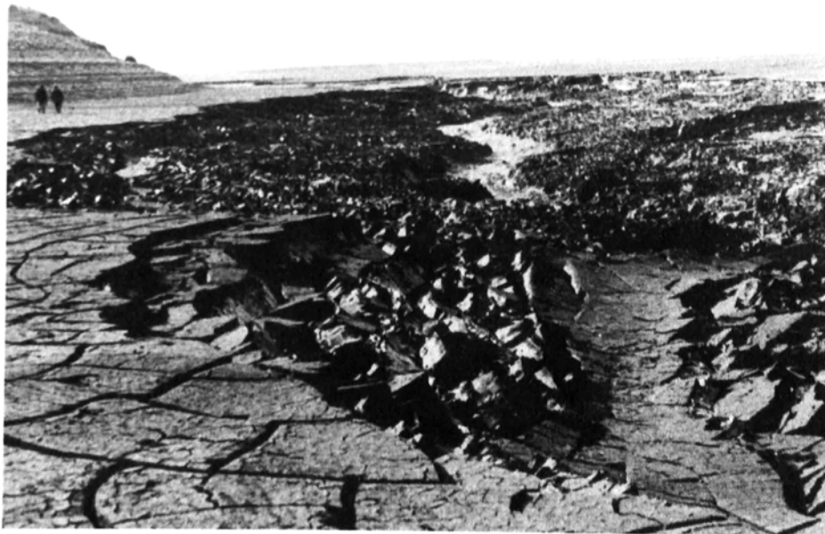
FIGURE 23.21 Slumping of poorly consolidated fine sediment in the lower reach of the longitudinal diversion channel ( E. Tolouie ).
