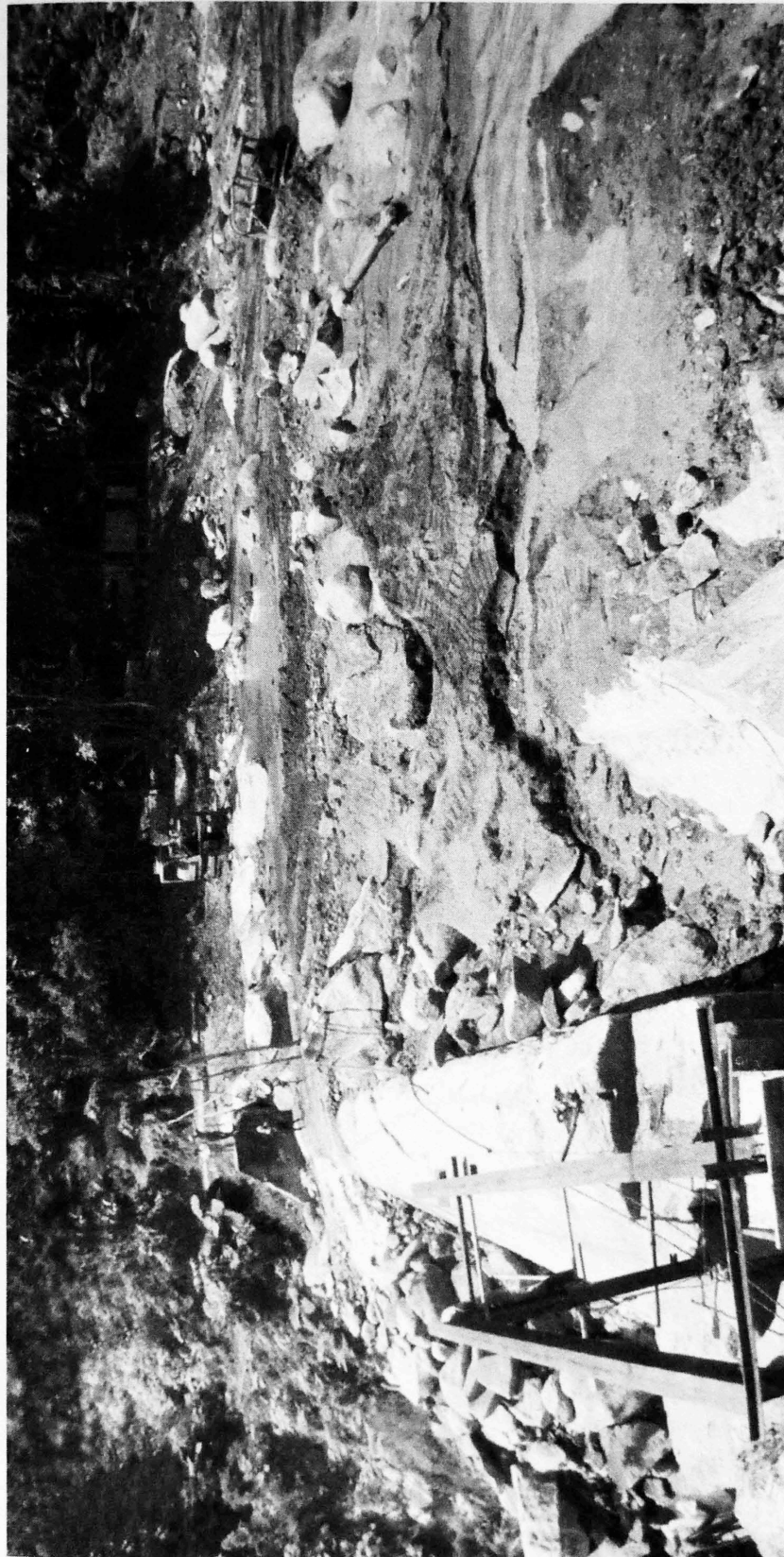
FIGURE 2.3 Hydropower diversion dam on Río Blanco filled with landslide sediment resulting from heavy rains during the passage of hurricanes David and Frederick through Puerto Rico in 1979 ( G. Morris ).
