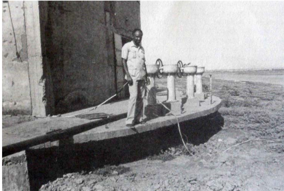
FIGURE 1.2 Sedimented water supply intake in the delta region upstream of Khasm El Girb a Dam on the Atbara River, Sudan ( R. Hotchkiss ).
