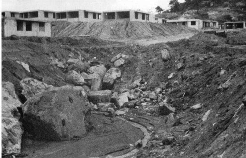
FIGURE 12.4 Eroding soil at a construction site in the watershed tributary to Loiza Reservoir. In addition to obvious sheet and rill erosion on bare slopes, the stream passing through the site has also been affected by earth movement. Although Puerto Rico has regulations requiring erosion and sediment control at construction sites, enforcement is lacking ( G. Morris ).
